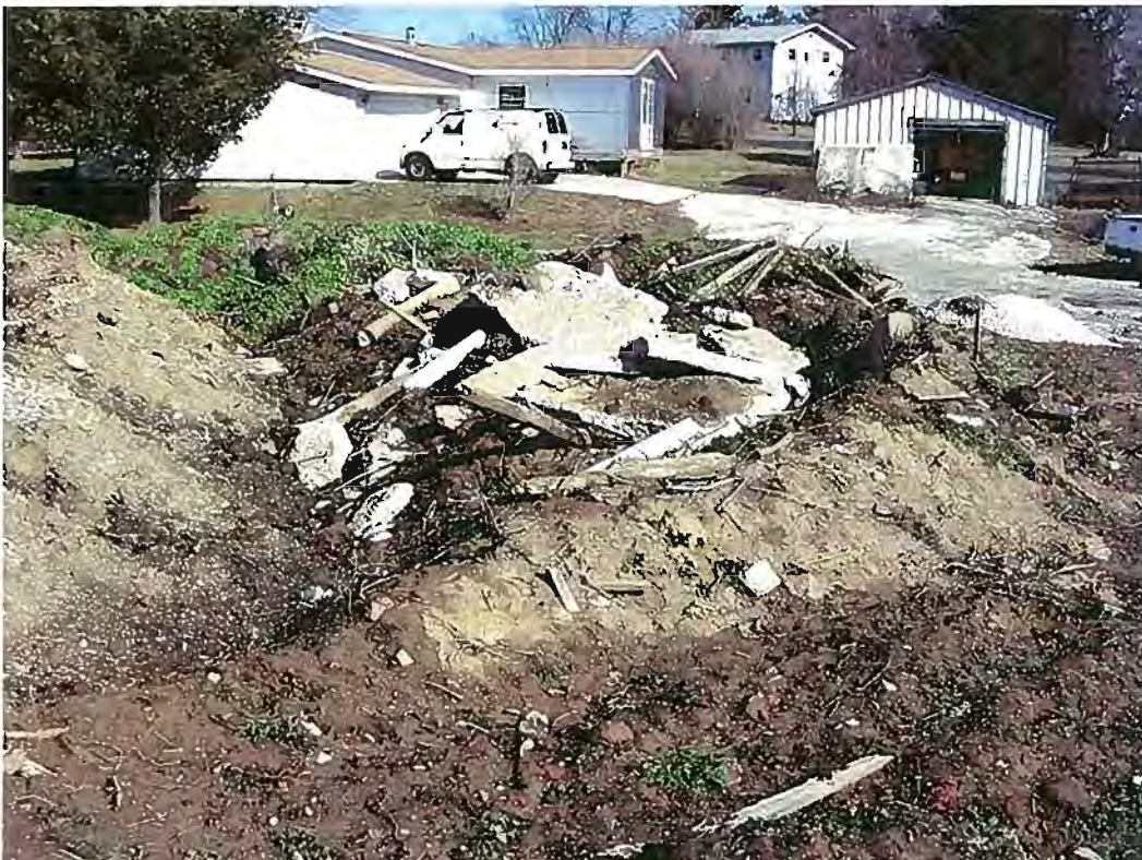
Date:01-30-2012 Time: 12:06PM Direction: Northeast Photo by: Jen O'Hearn Exposure #: 010 Comments: View of dimensional lumber and concrete in with dirt pile and dimensional lumber on ground. At rear of photo rebar visible as seen in photo #3.
